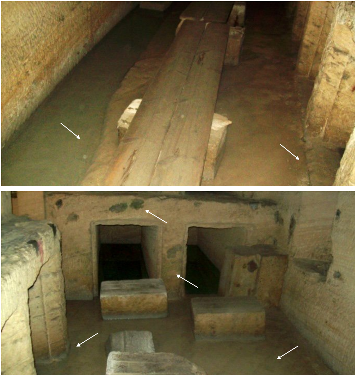
Figure 3. Presence of groundwater in the third level of the Catacomb tombs and its influence at the walls: algae growth and deterioration of plaster and limestone.
